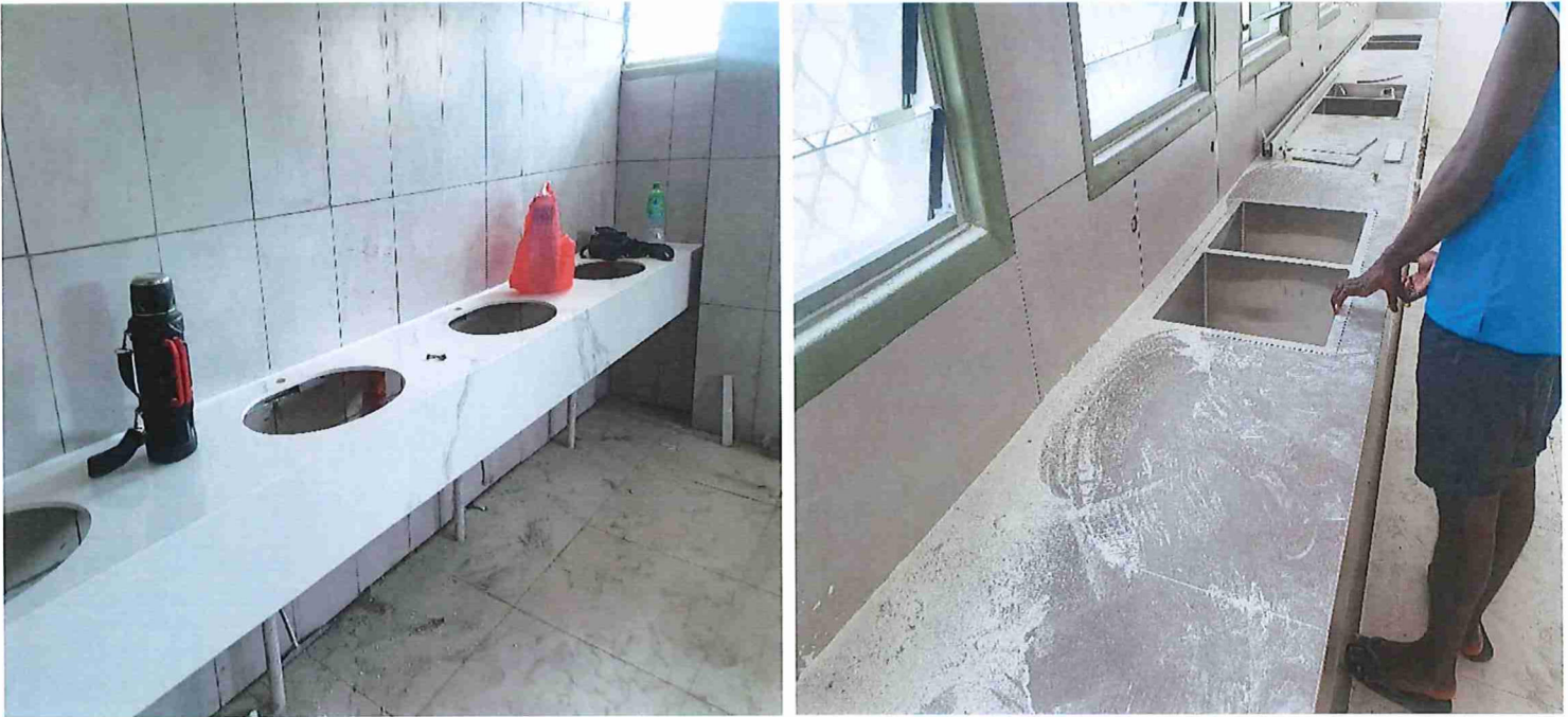
Figure 9. hand wash section – ablution & Laundry area (B/F)
