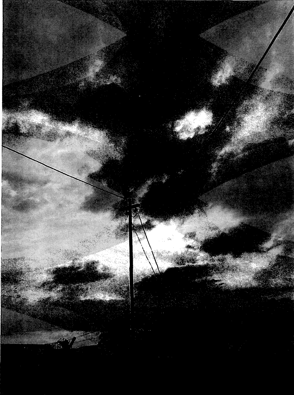
Figure 1 Service line complete installation for supply connection to building 6.
