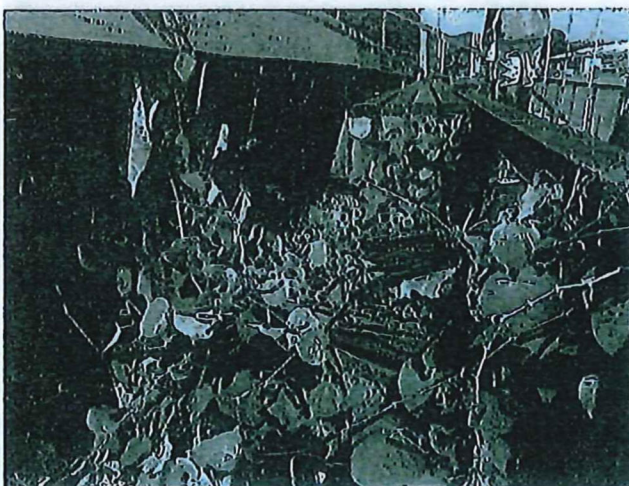
Figure 10: Southeast stands- damaged sitting floor tread
