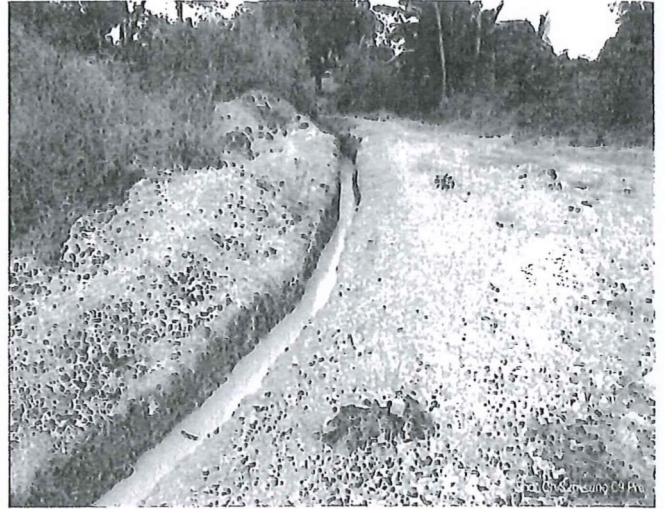
Figure 2- Drainage diverted from the existing and proposed Drainage route at chainage 390.00m
